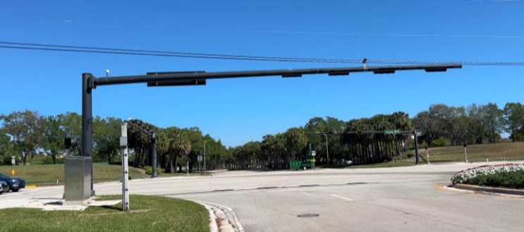
Sunrise / NW 136 Ave Fiber Optic Network
