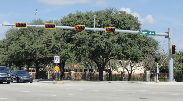
Stirling Road & Palm Avenue Mast Arm
