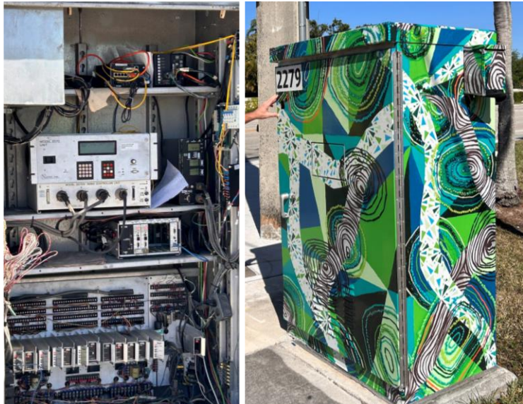
Pine Island Road Fiber Optic Network
