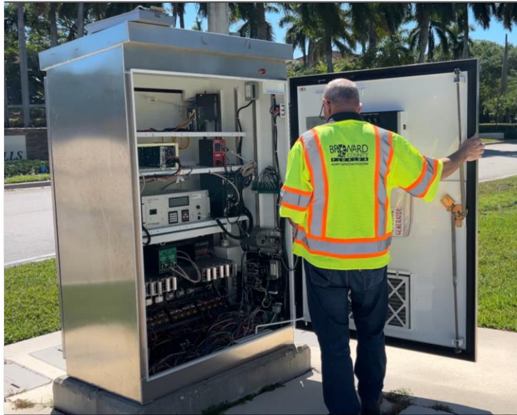
Sunrise / NW 136 Ave Fiber Optic Network
